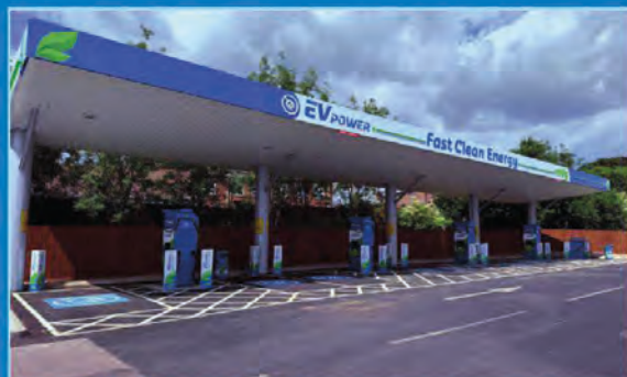
400 kWh EV Charging Hub
