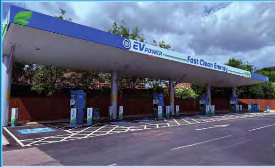
400 kWh EV Charging Hub
